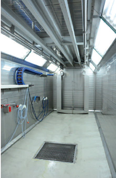
The pre-treatment of the aluminium parts includes the following process steps: pickling/degreasing, washing 1, washing 2, de-mineralised washing and passivating.
